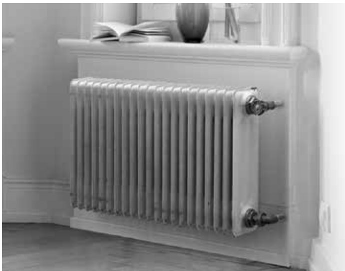
Before: Old radiator
